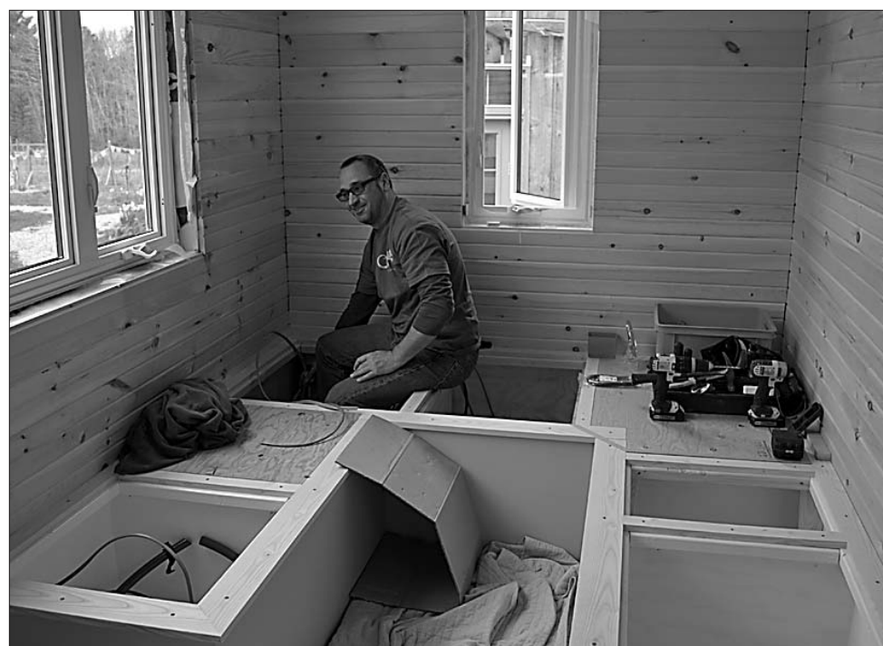
Kuno Kuenzle of Green-Lizard Energy Solutions works at installing equipment to run the off-grid power supply to the unit currently being built for Dawn Higgins.
