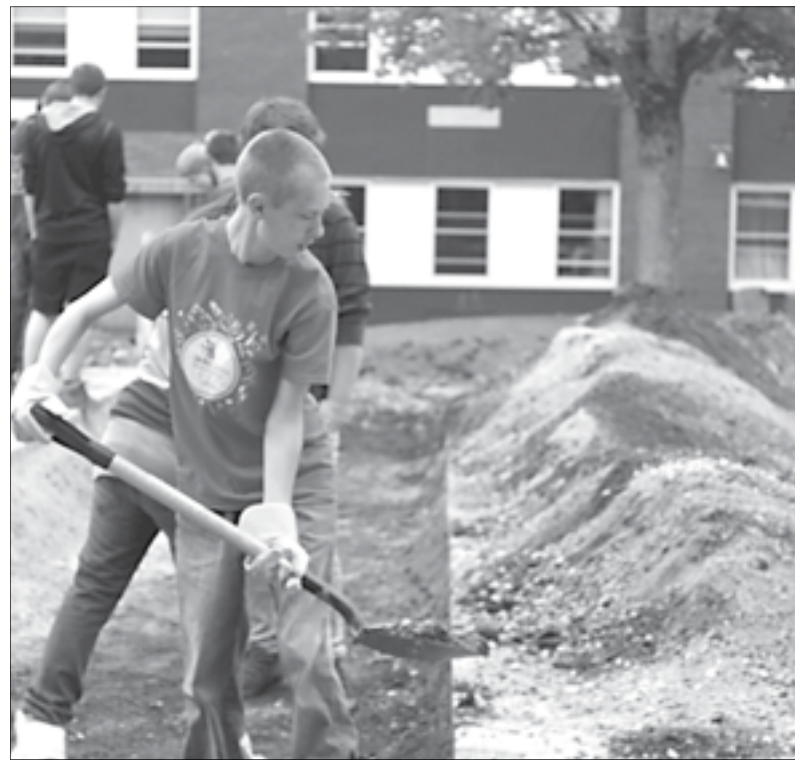
Grade 10 student Cyle Legacy works on Bridgewater Junior Senior High School’s green space on June 5.
